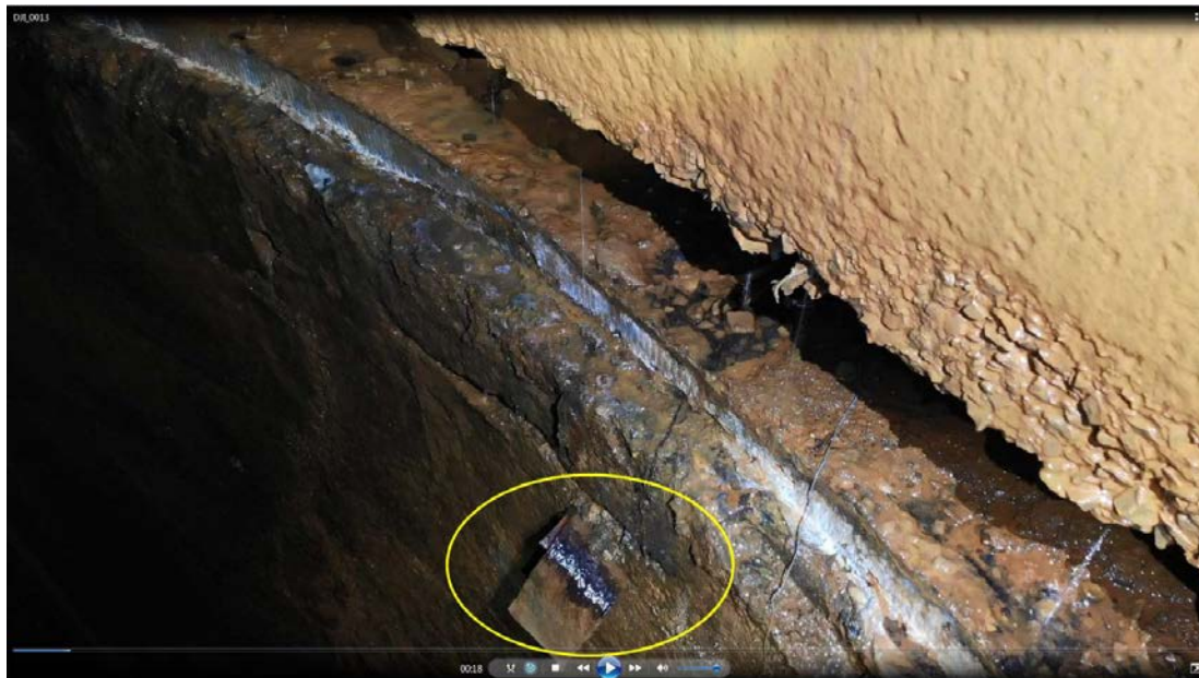
Photograph 2: Water ring bracket damage in shaft. Photograph by Resources Regulator
