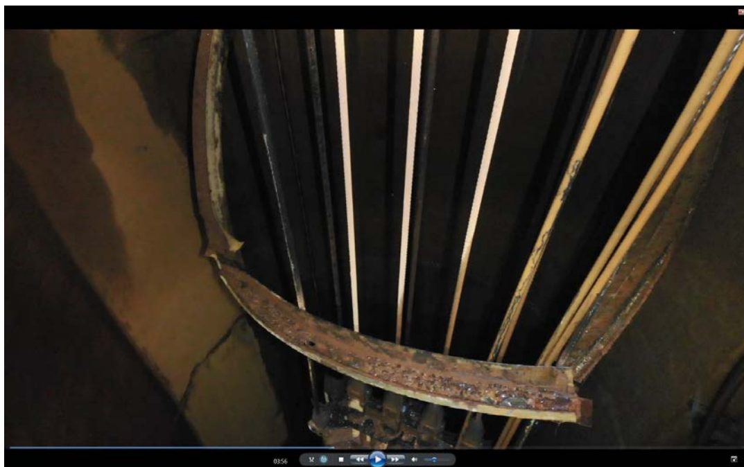
Photograph 3: Water ring wrapped around guide ropes, head ropes and services in shaft. Photograph by Resources Regulator
