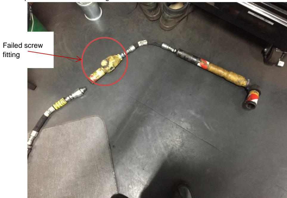
Figure 1 – photo of failed screw fitting
