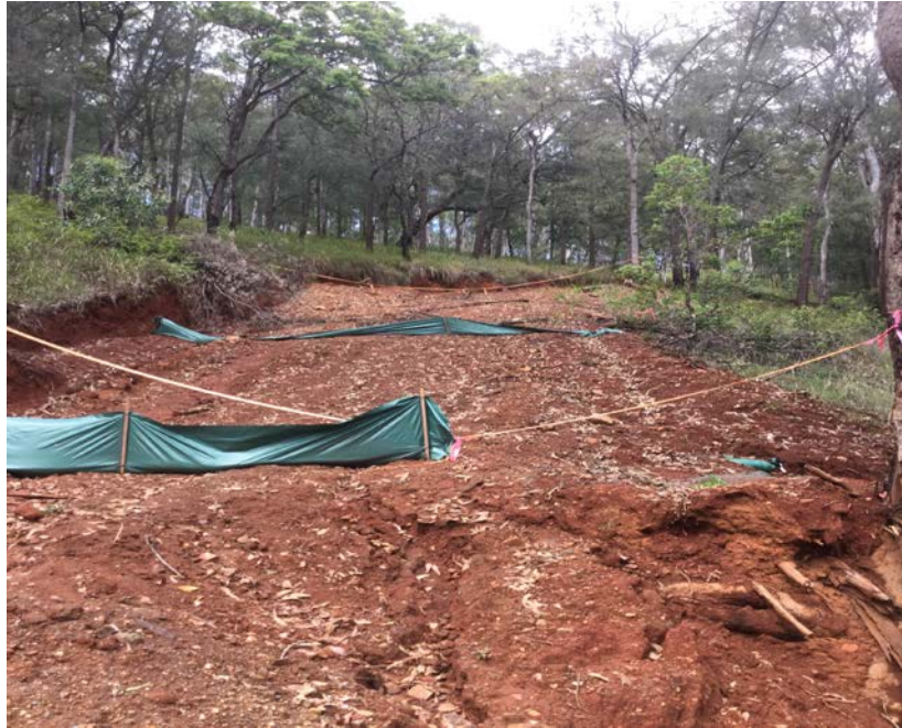
Figure 1 Inadequate sediment and erosion controls
