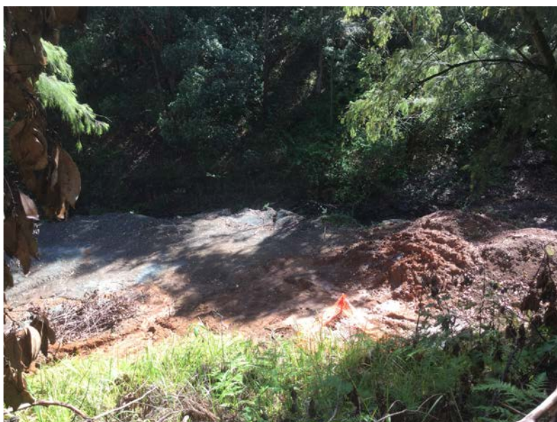
Figure 2 Poor drill cutting management and substandard erosion and sediment controls near a watercourse
