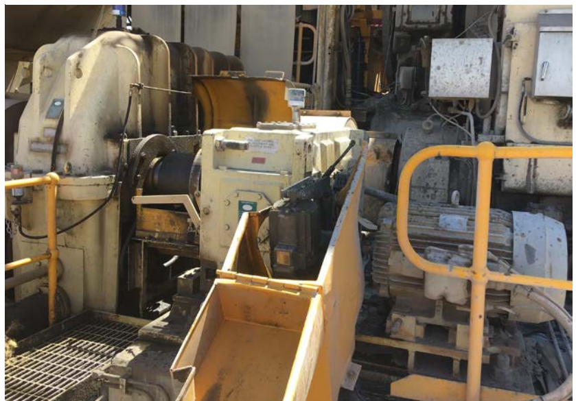
Figure 1 The drive assembly showing two gearboxes (left and right), motor and failed brake assembly
